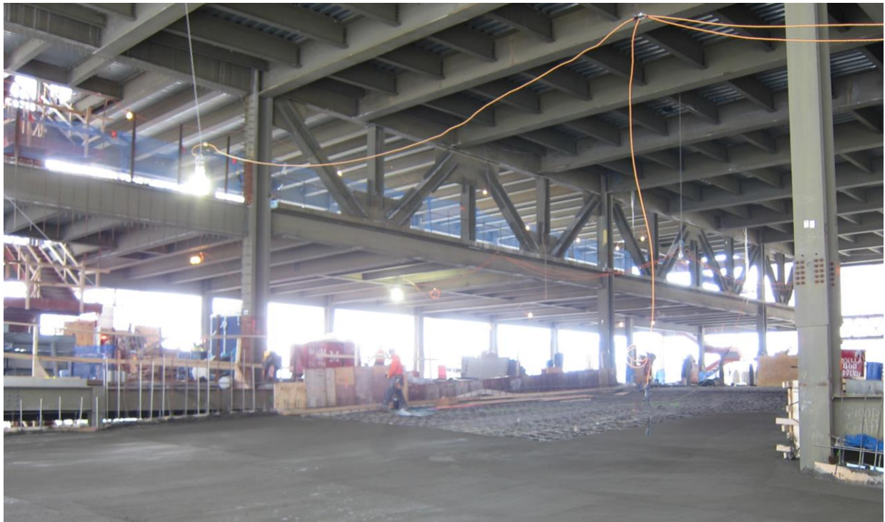
Image No. 6 - View of the full floor height trusses along Column Line 2 designed to support the personnel floor and the truck floor.
