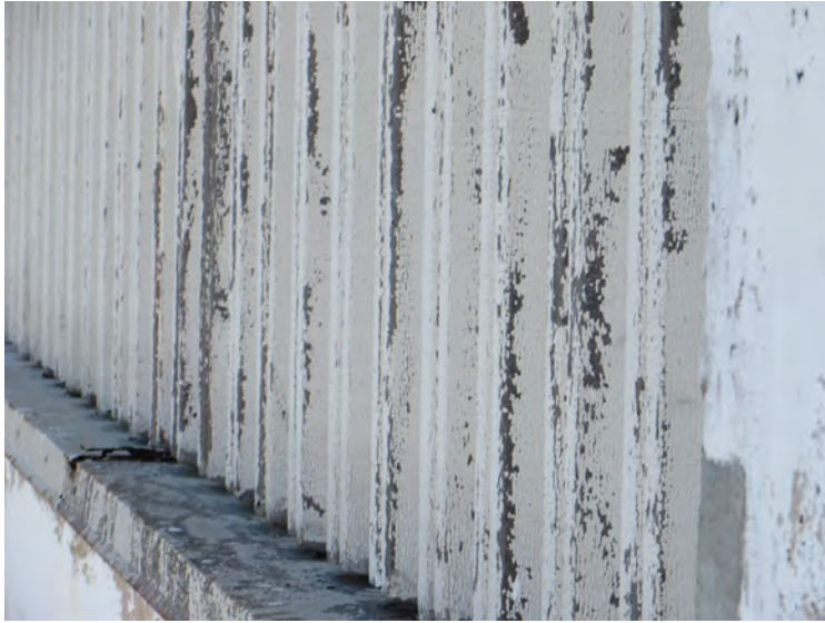
BEFORE: General condition of facade before repair
