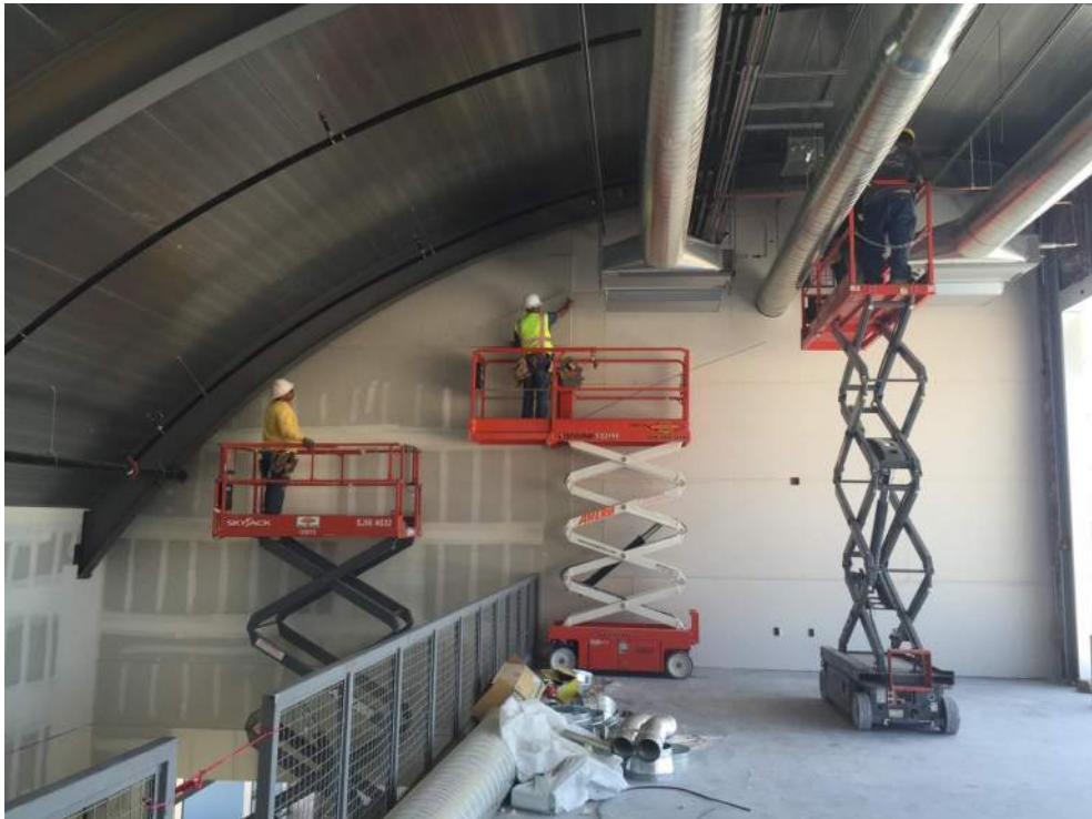
Exhibit F (Below): Contractors work on the interior fit-out during the final phases of construction. Note the curved HSS beams at the top of the photo and clear space to below.
