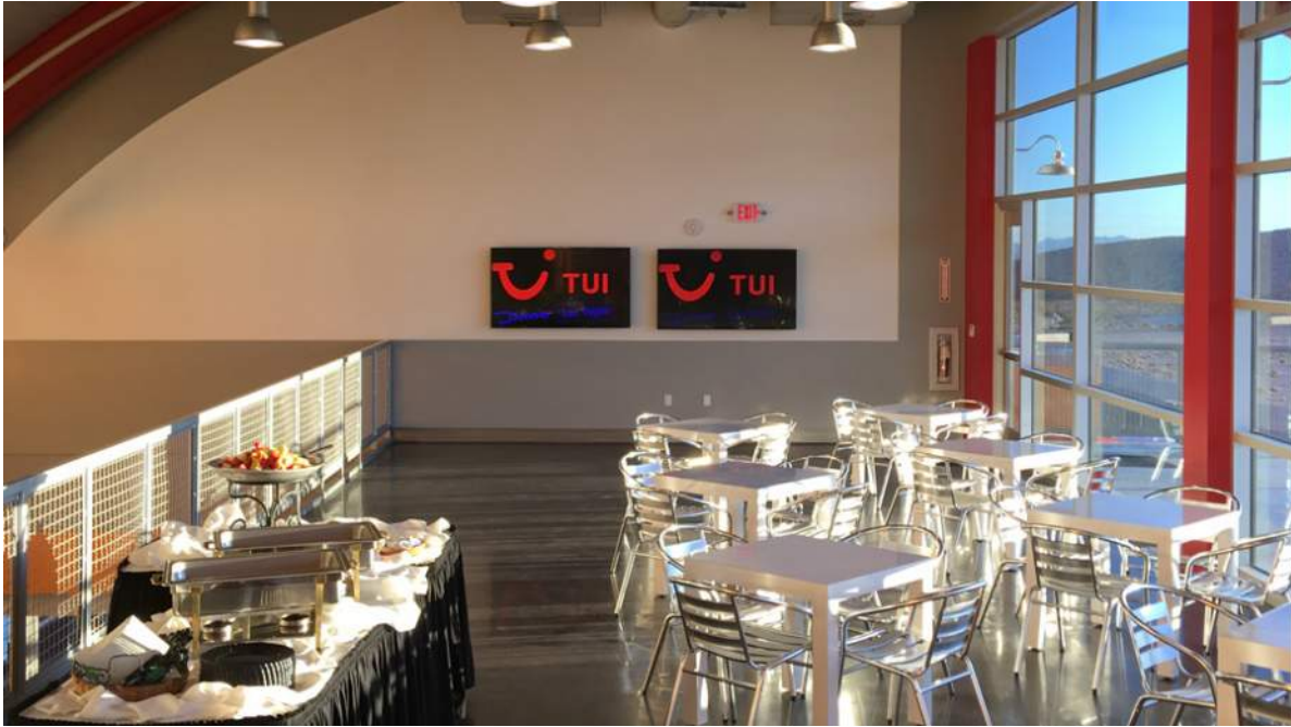
Exhibit E (Above): Arrangement of second level showing the column-free space, arc of the HSS beam supporting the roof. Note that the second level opens to the ground-level below.
