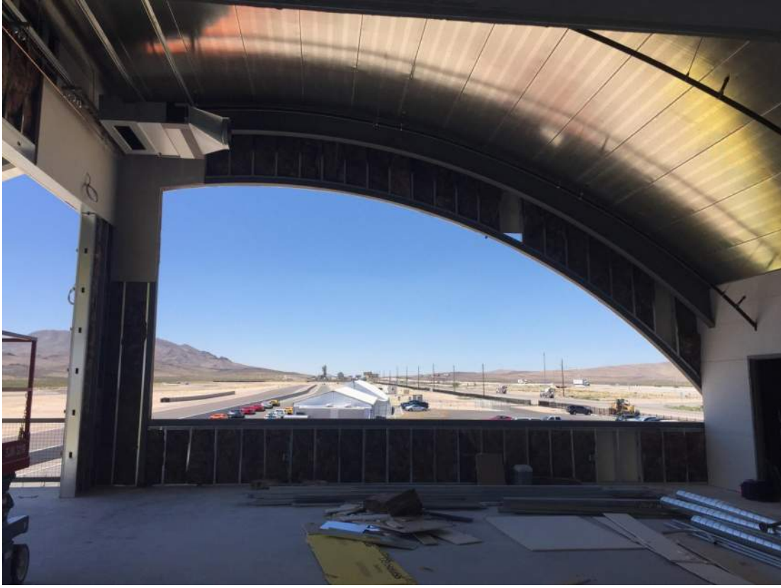
Exhibit H (Below): Contractors work on the interior fit-out during the final phases of construction. Note the curved HSS beams at the top of the photo and clear space to below.
