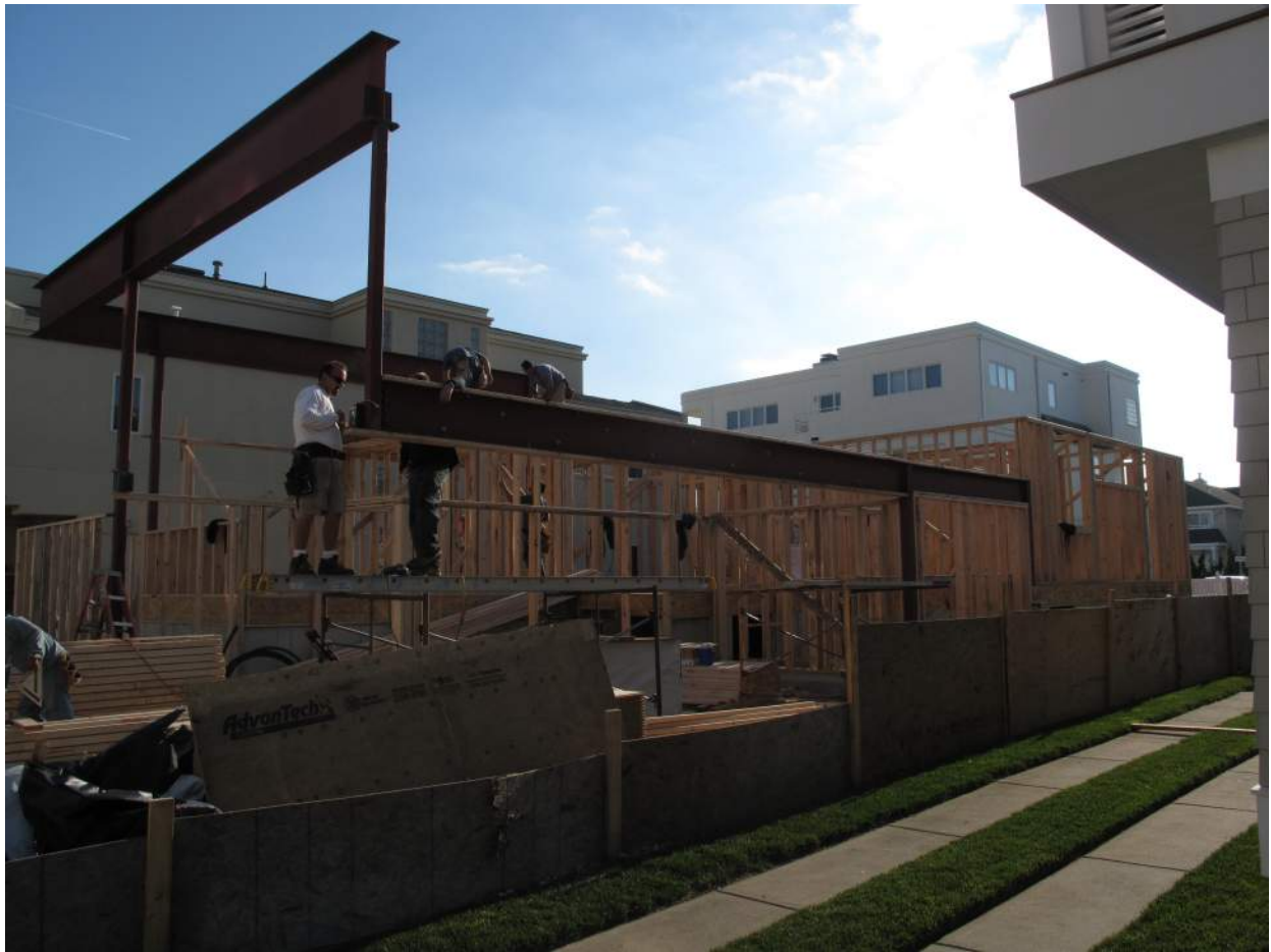
Exhibit E (Above): Contractor checks level for WF beam for suspended floor support over garage space. Note that the transfer girder framing for the master bedroom is suspended by hanger from an additional transfer girder above. The far beam is a W24x62 supported by HSS columns.
