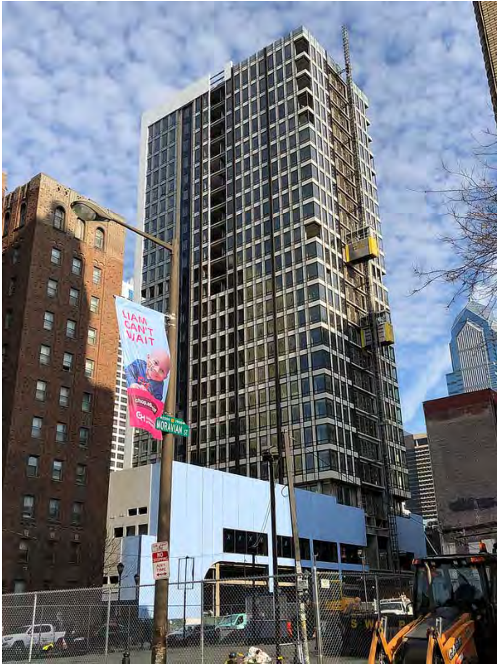
The Harper with tower façade almost complete. Scheduled to open to residents on 6/1/2019.
