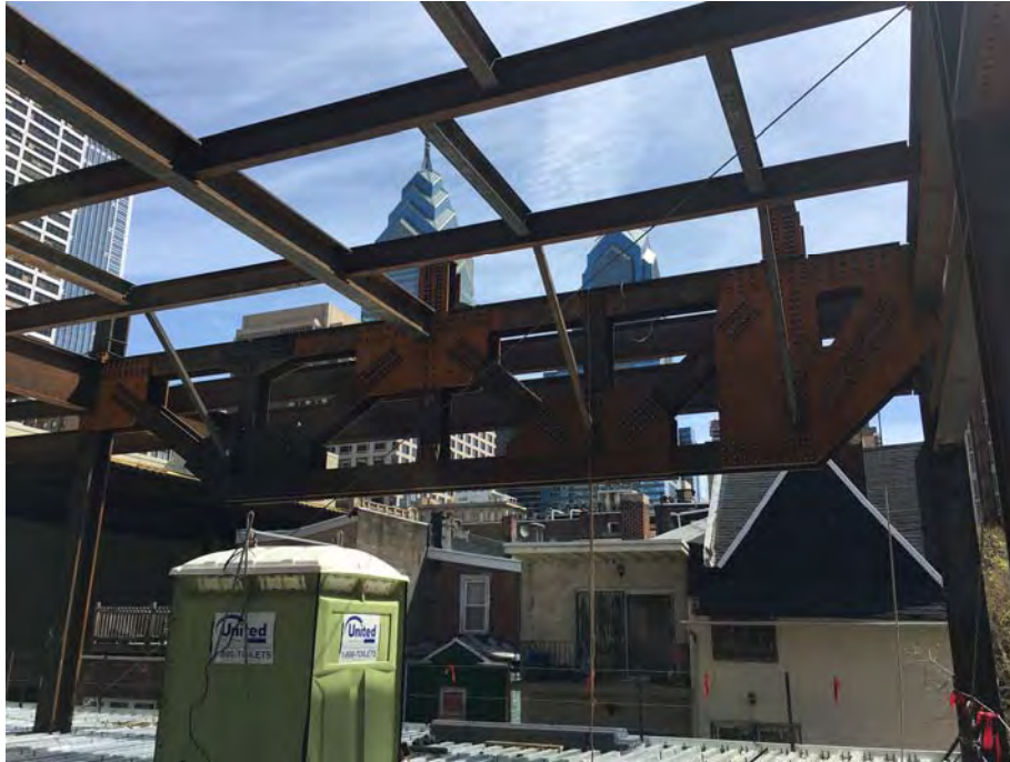
Transfer truss showing nodal bracing of the compression web members.
