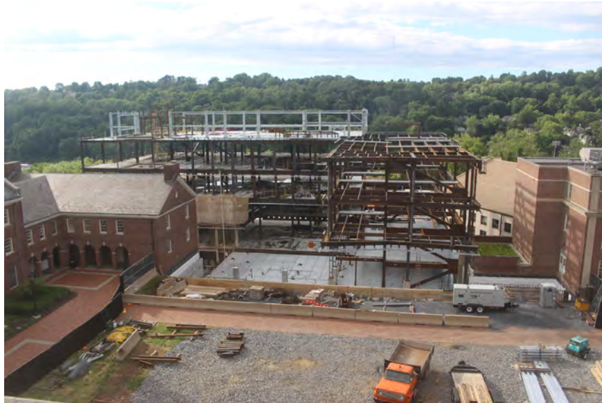
Steel superstructure erected with formwork for 16" cast-in-place concrete slab to support courtyard extension on to building
