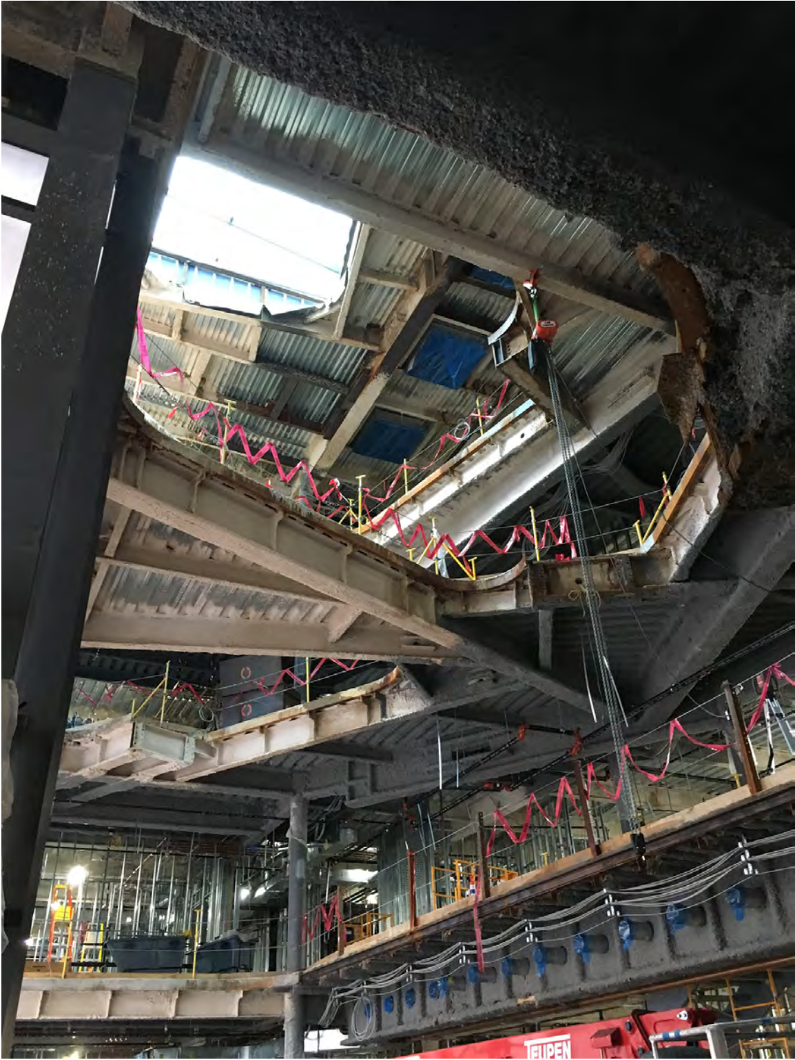
Complex atrium framing forming organically shaped floor openings, sized for vibration control of the atrium stairs, and showing beam web openings.
