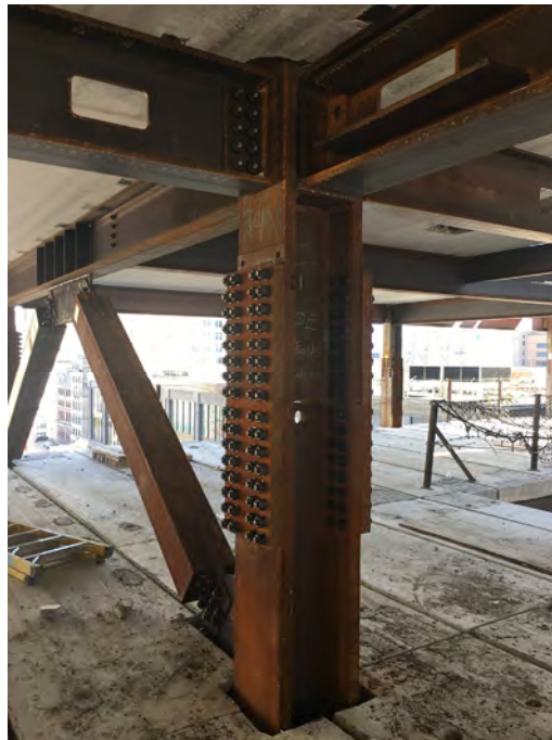
Phase 2 braced frame column splice at the 4 th floor. Note beam penetrations for getting utilities into the units.
