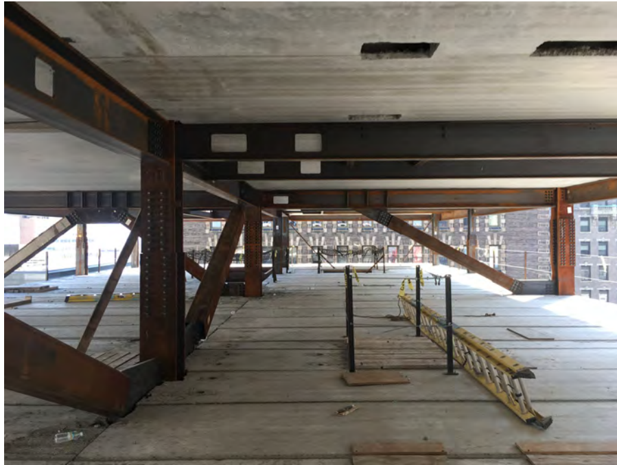
Phase 2 – Note eccentric braced frame to accommodate the central corridor as well as the beam penetrations to allow utilities to run in the corridors.
