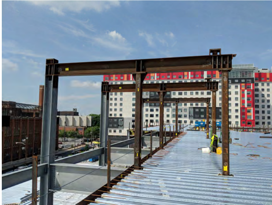
6 th Floor Level Transfer Framing above 5 th Floor Primary Transfer Level with exposed columns against curtainwall façade
