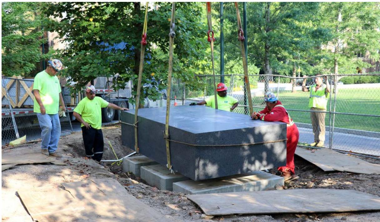
Nevelson sculpture and Nevelson base. Note the slots in the concrete foundation of the base, which were included to accommodate the rigging used to lower the base on to the new foundation.
