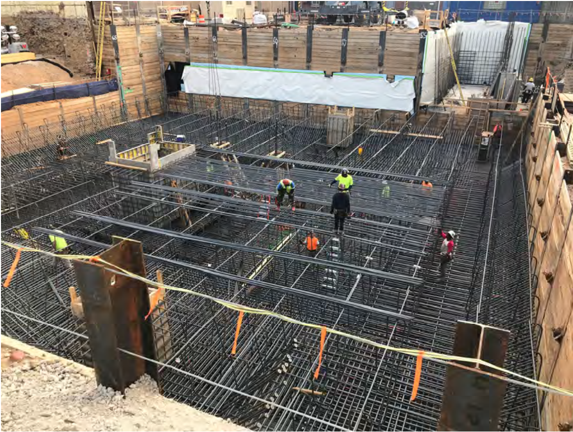
Top reinforcement under way for the 12' and 8' thick mat foundation. Bottom mat of reinforcement already placed.
