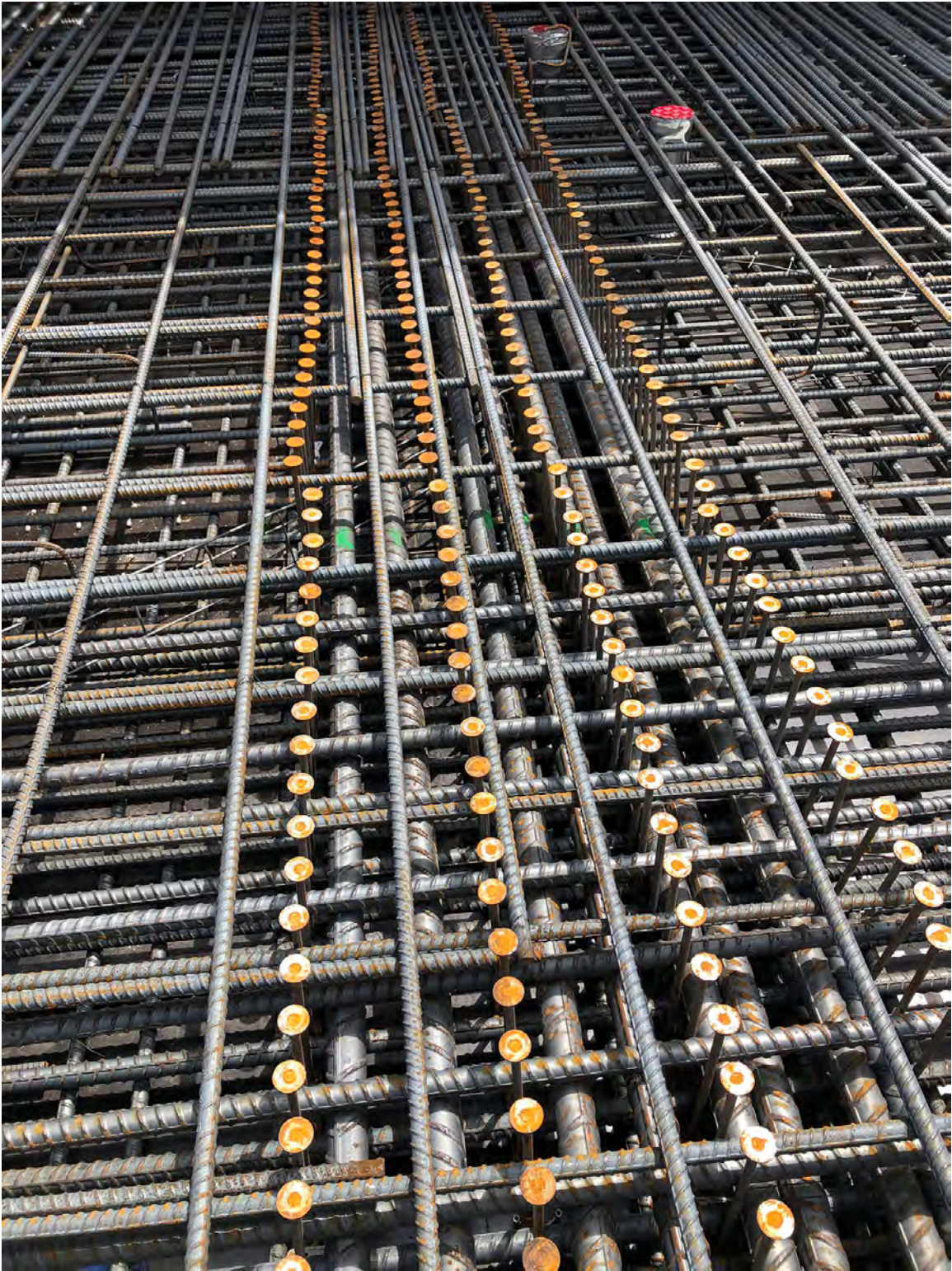
#18 bars and stud rails for tension forces at 8 th floor from walking columns
