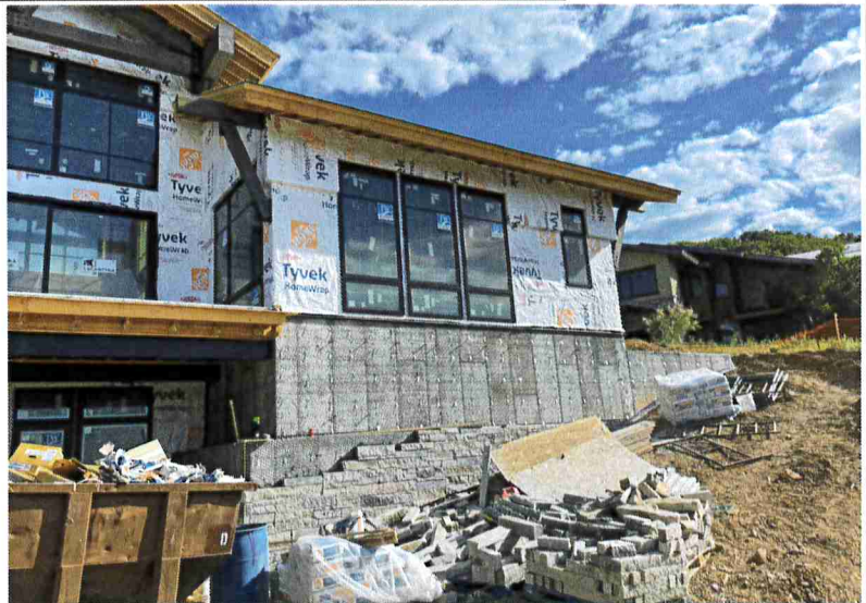
STEPPED FOUNDATION WALLS TRANSITIONING FROM HIGH CRAWLSPACE TO BASEMENT SLAB ON GRADE TO RECEIVE STONE VENEER
