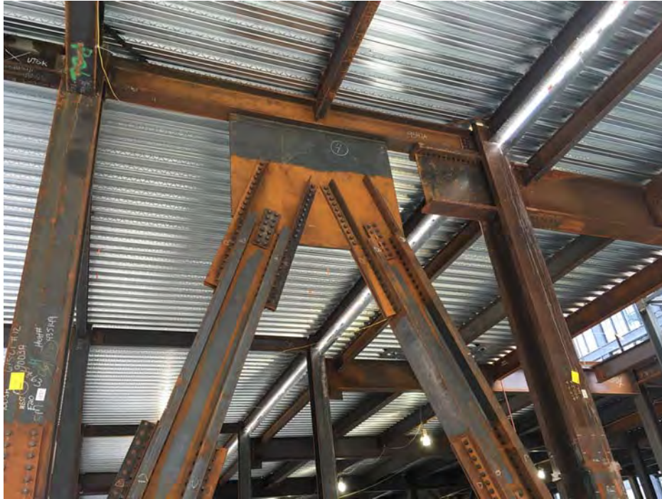
Phase 1 Braced frame with lateral drag connection shown on the upper right to transfer lateral forces from the tower to the podium.
