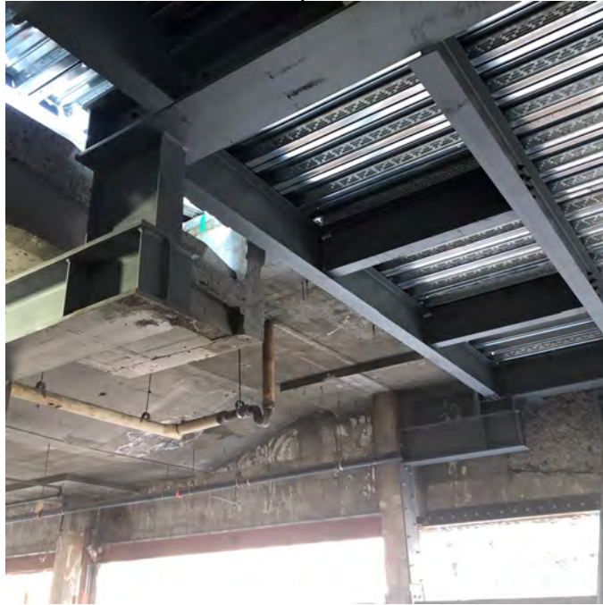
New bent steel to support terrace, accommodating varying heights of existing structural elevations.
